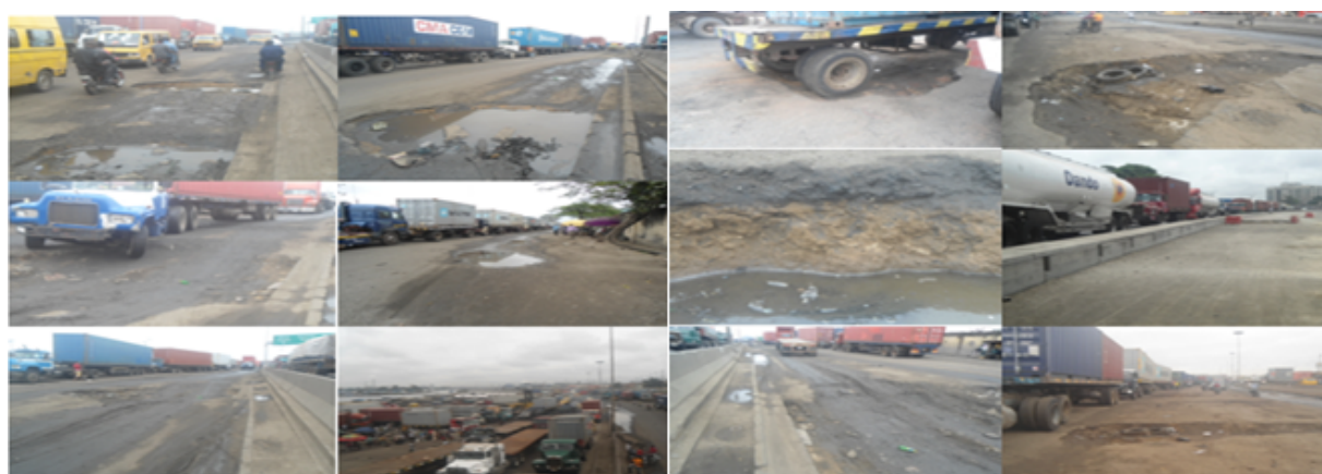
Figure 4: Damages caused by overloaded trucks thereby exerting pressure on the road pavement. This is the major reason for pavement damage along Apapa traffic corridor where about 16-25% of the traffic is mainly heavy duty trucks, trailers, oil tankers and container trucks.
